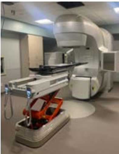
Radiation Oncology Center's renovated vault and new linear accelerator
